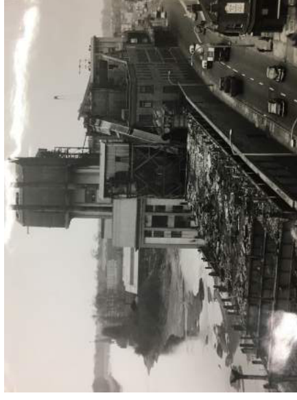
Demolition in progress the bank of purifiers are in the foreground – 1965 Finished in October 1966
